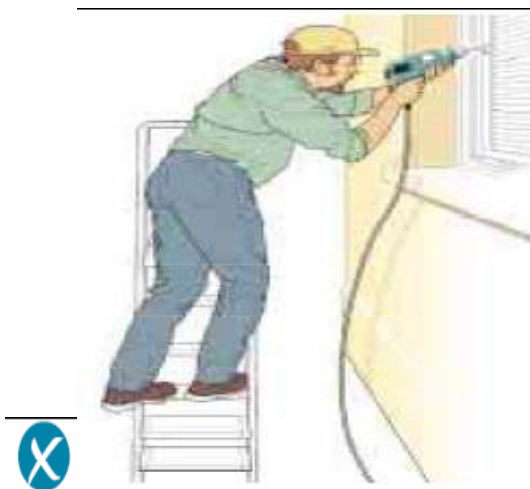
Incorrect – steps side on to work activity
