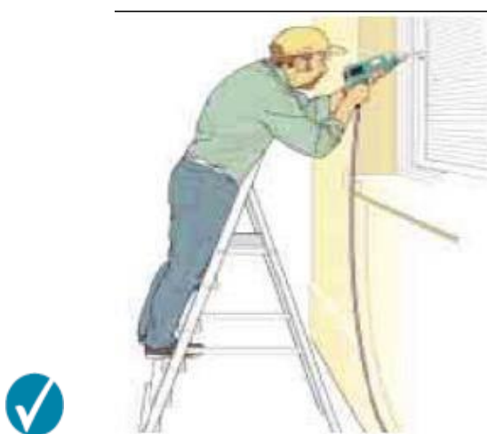
Correct – steps facing work activity
